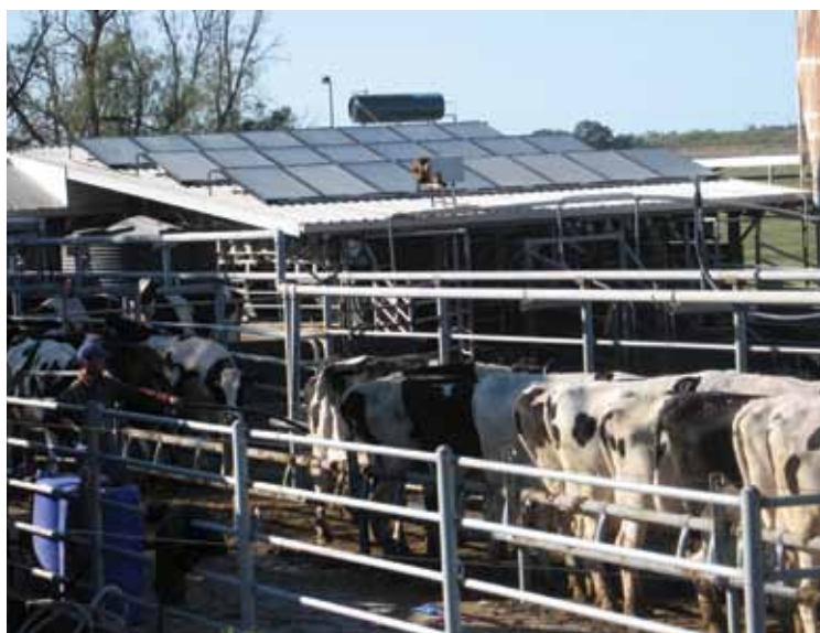
The solar system saves about 183.3 kW a day or 36 tonnes of CO 2 a year.
