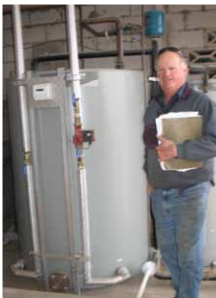
When moving to solar power, Ray Dohnt opted to install a larger (2,500 L) storage tank in case their needs increase in the future.
